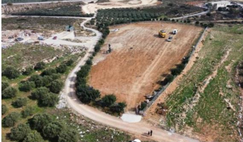
Virtual net-metering PV project (405kWp) located at Sarafali Mandra
